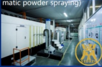
Reciprocating machine (automatic powder spraying)
